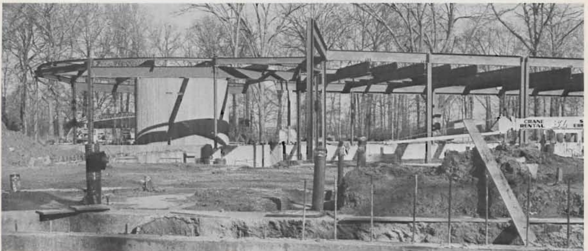
Construction of the new Primate and Feline Building continues as workmen are now setting the steel to form the walls. The building is scheduled to be completed in 1977 and will then house the Zoo’s ape and cat collection.
